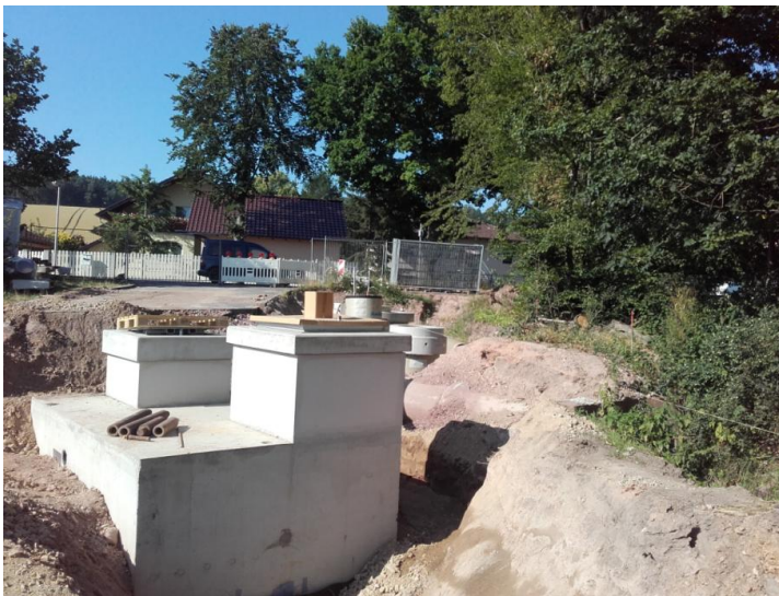
Pumpstation Hecke Ost
